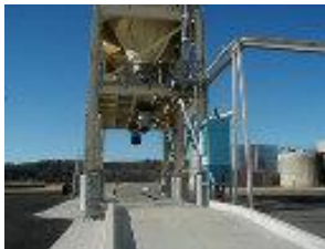
Storage silos used to temporarily store dried pellets on-site.
