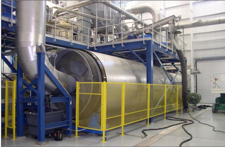
Heat Dryer System at SCWRF
