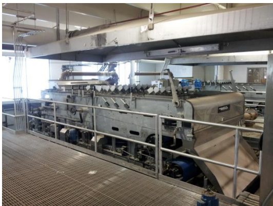
Combination thickening and dewatering belt filter press at WWRWRF
