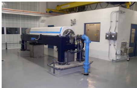
One of two centrifuge dewatering units at SCWRF
