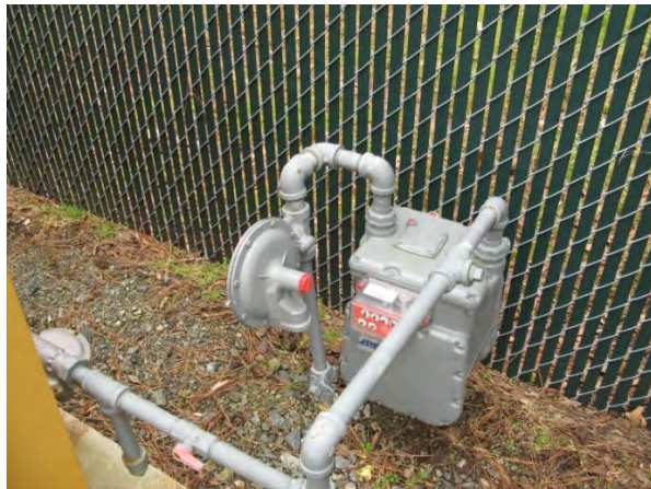
Generator Gas Line
