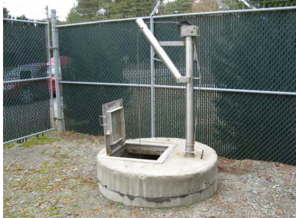
Basket Vault & Crane
