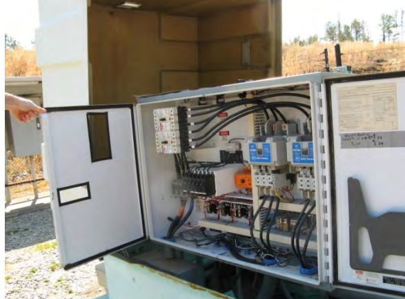
Pump Control Panel
