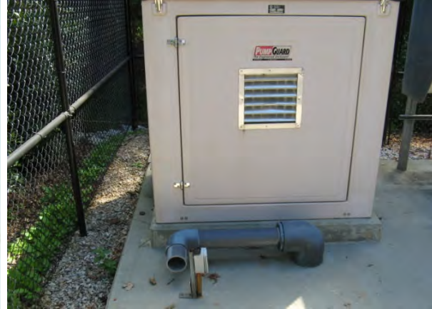
Grinder Hydraulic Unit
