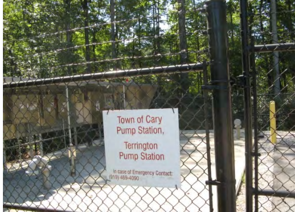
Terrington Pump Station
