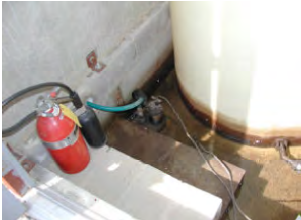
Odor Control Chemical Containment
