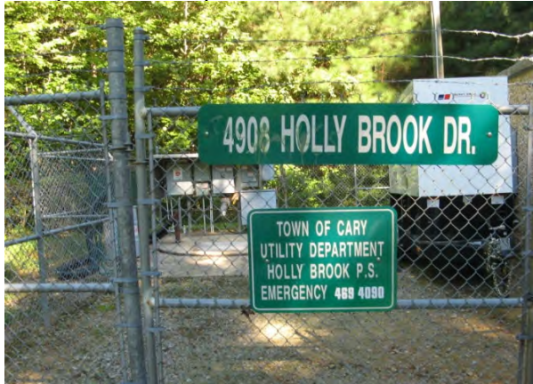
Holly Brook Pump Station
