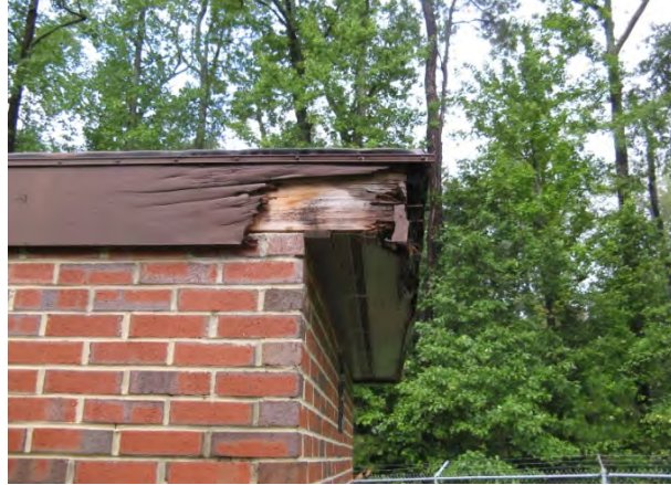
Fieldstone Pump Station
