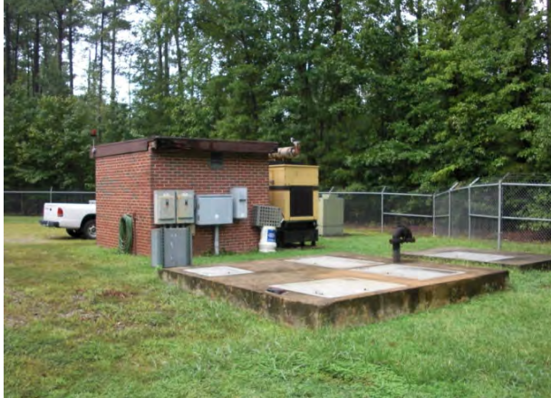
Fieldstone Pump Station
