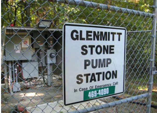
Glenmitt Stone Pump Station
