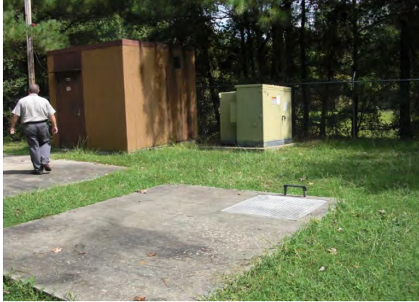
Nelson Road Pump Station
