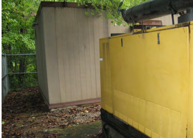
Generator & Chemical Building
