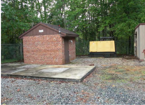
White Oak Pump Station
