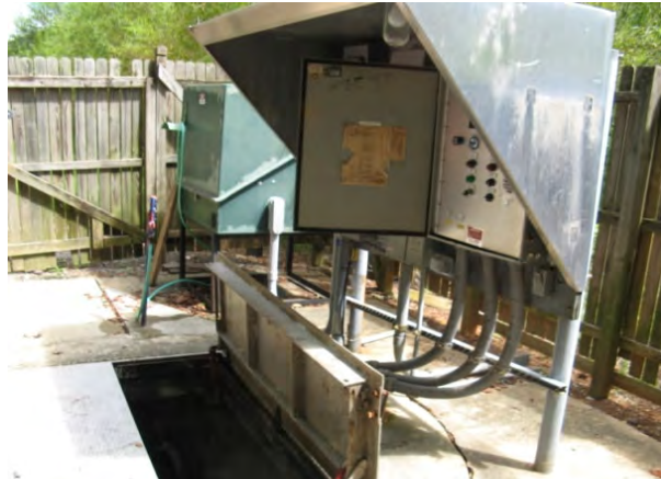
Wetwell and Control Panel
