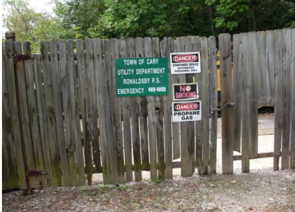
Ronaldsby Drive Pump Station
