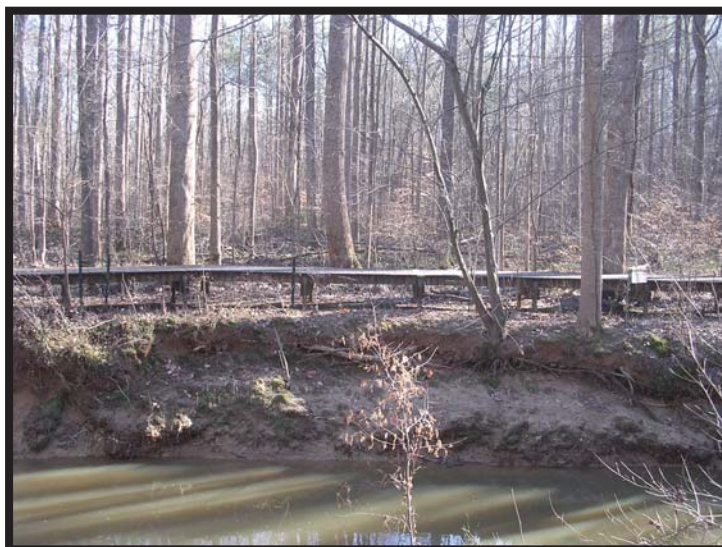
View across the creek looking at the boardwalk & eroding streambank
